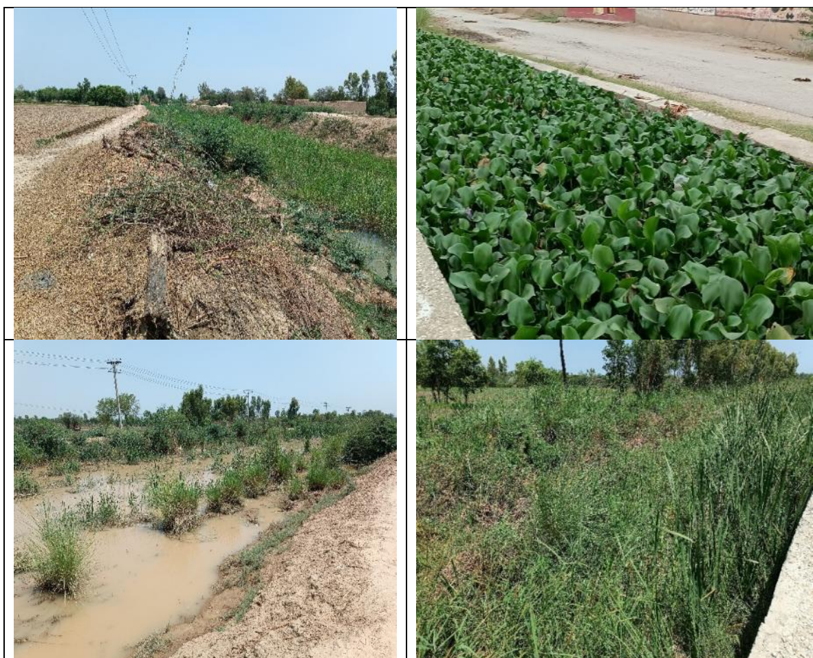
Figure 2.1: Heavy Silt, Vegetation and Sarkanda in Drains
